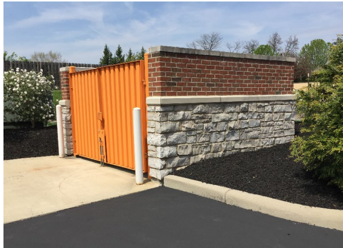
Figure 6.3-1: Dumpster enclosures, whether attached or not attached to the principal structure, shall be constructed of brick and/or natural style stone material.
