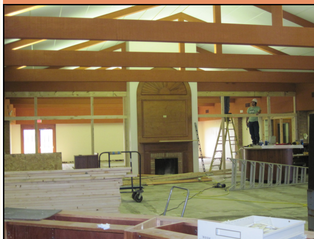
Photo at left shows the Lakota Area Activity Center under construction. The Center is planning a Fall opening.
